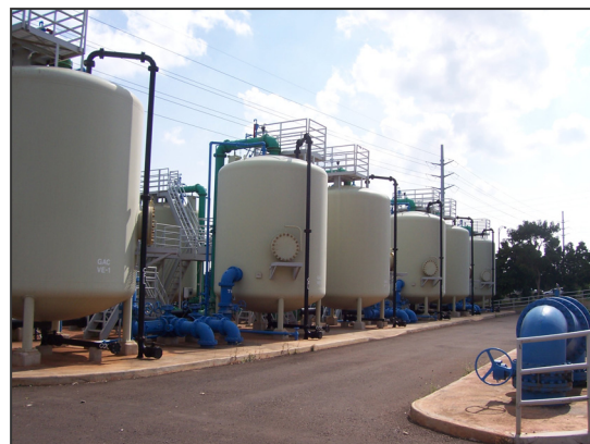
Kunia Wells I treatment facilities.
