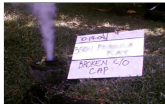
Broken cleanout cap, a source of infiltration / inflow.
