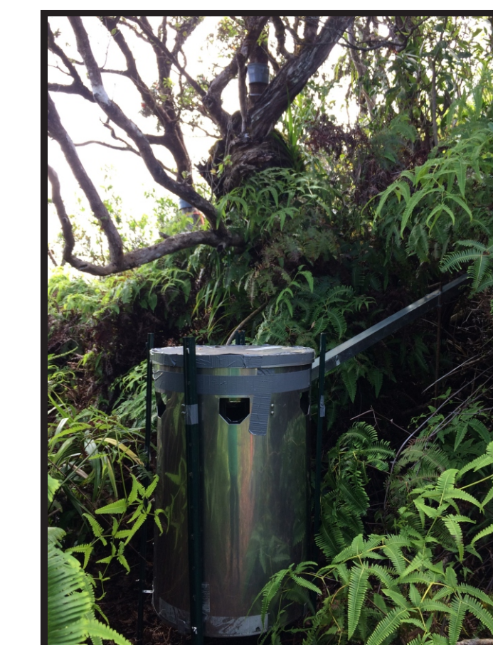
Throughfall Equipment: For each test plot, a total of three troughs lead to a fabricated tipping bucket (150 mL / tip) rain gauge. The gauge is nested in a stainless steel can, levelled and anchored to the ground for stability. Troughs were installed under trees typical of the test plots (species, diameter, height) in configurations that represented the average canopy and gap proportions and minimized overlap of throughfall collection between troughs.
