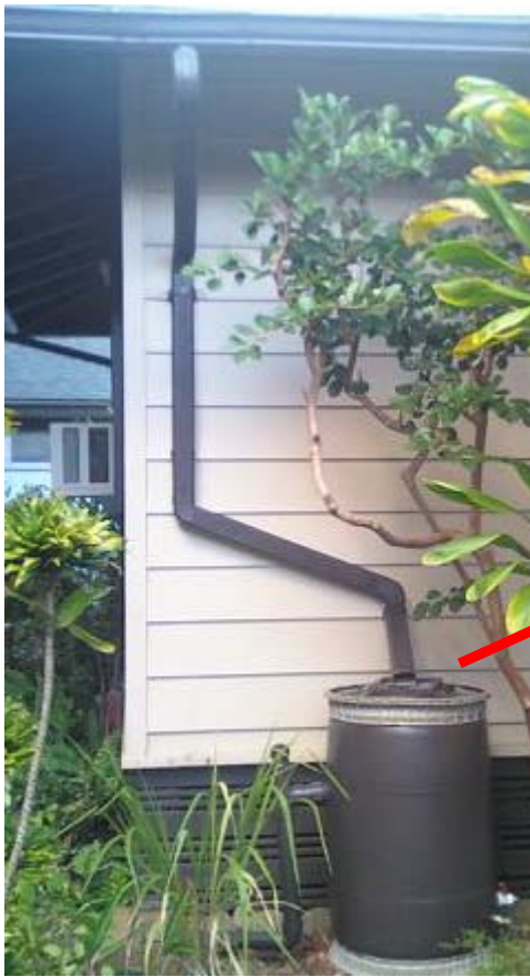
Screen and wire mesh secured over opening from downspout to capture debris from roof. Screen secured over existing openings.
