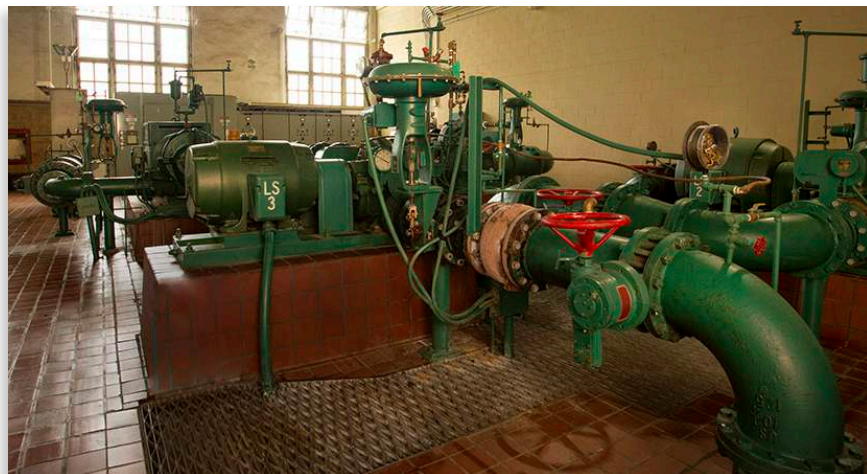
The BWS wells and pump stations can be found both outdoors and indoors.
