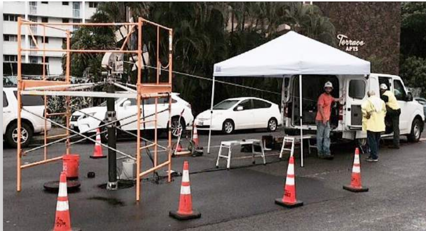
Advanced pipeline condition assessment requires traffic control, excavation, construction of a vault, tapping into water-filled pressurized pipe, and installation of a valve. The testing team tracks a probe inserted into the pipeline, propelled by the moving flow of water, up to a distance of ½ mile.
