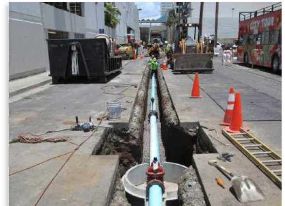
Recommended future pipeline construction includes installation of new pipes as well as renewing and/or replacing existing pipes.
