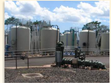
Granular activated carbon treatment facilities remove legacy agricultural contaminants from the drinking water supply in Central O'ahu and 'Ewa-Waipahu.
