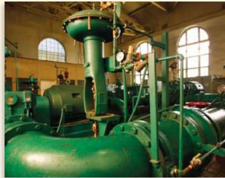
Pumps at the BWS Beretania Pump Station extract water from underground aquifers and move it to reservoirs in the area.
